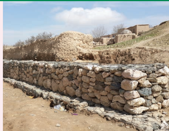
Gabions are walls that are constructed by filling large galvanized steel baskets with rocks, which helps to block floodwater and debris from landslides, reducing the effects of natural disasters.
